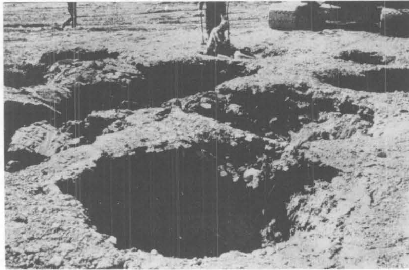
Figure 23. Ground heave induced by dynamic compaction.
